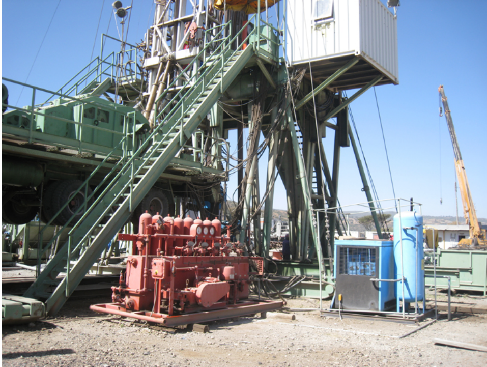
Photo 6: Blow Out Preventer Activator
