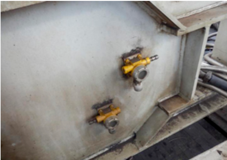
Hydrogen sulphide sensor installed but not connected.
